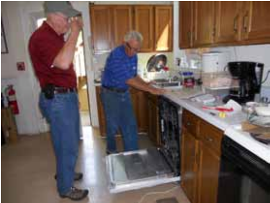
Drew Sampson & Roy Millar installing a new dishwasher in Brooks Hall as part of our transition.
